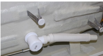
Easy Clean Bath Waste fitted to a freestanding bath with flexible pipe fitted
